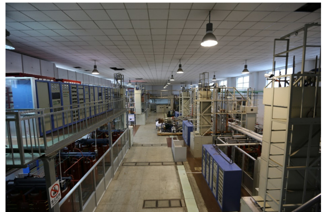
Fig. 2. View of 12.0 ICRH system in EAST ICRF hall.
