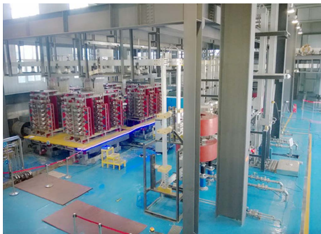
Fig. 5. Photograph of an 80-kA PS system.
