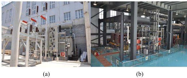
Fig. 19. Integration test of the PFCU prototype at ASIPP site. (a) Outside prototype. (b) Inside prototype.
