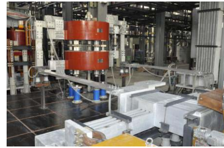
Fig. 17. Type tests site of the dc reactor at ASIPP site.
